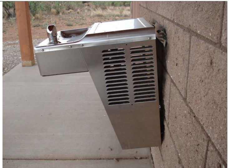
Water Fountain pulled away from Bathroom Facility
