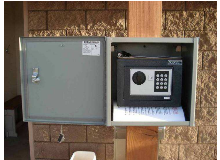
Combination Key Safe Mounted in the Enclosure
