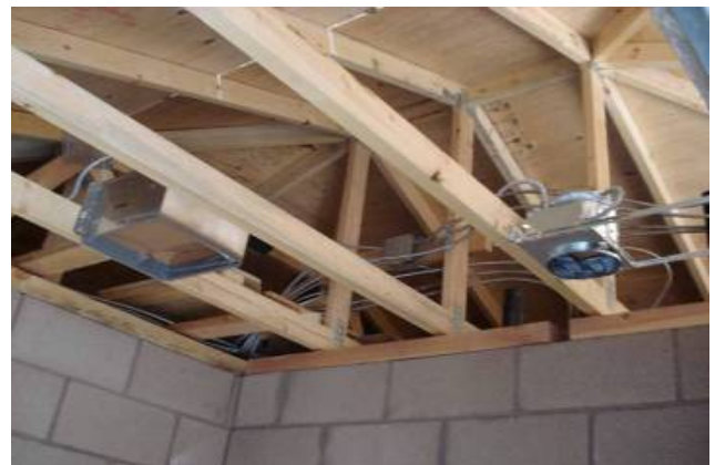
Bathroom Facility – Exhaust vent & interior lighting fixture
