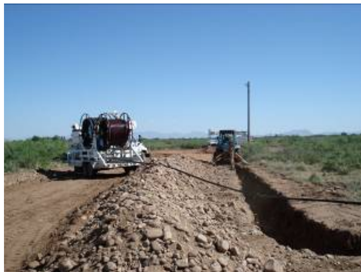
Primary electric power trench along entry road
